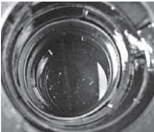
1. View of the shaft without filter.
